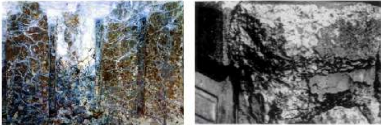
Figure 4. Concrete element after freeze-thaw cycles [7]
